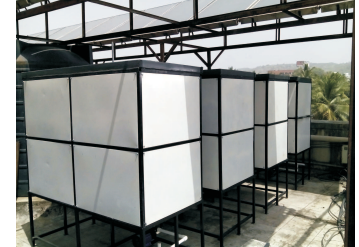
External Site Insulated Tanks
